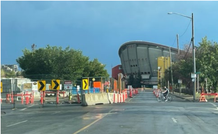
Looking south at deep utility relocation work along 12 Avenue S.E., between 6 Street and 5 Street S.E.
