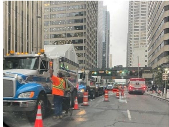
Looking east at Calgary District Heating Inc. pipeline relocation work along 5 Avenue S.W., west of 2 Street S.W.
